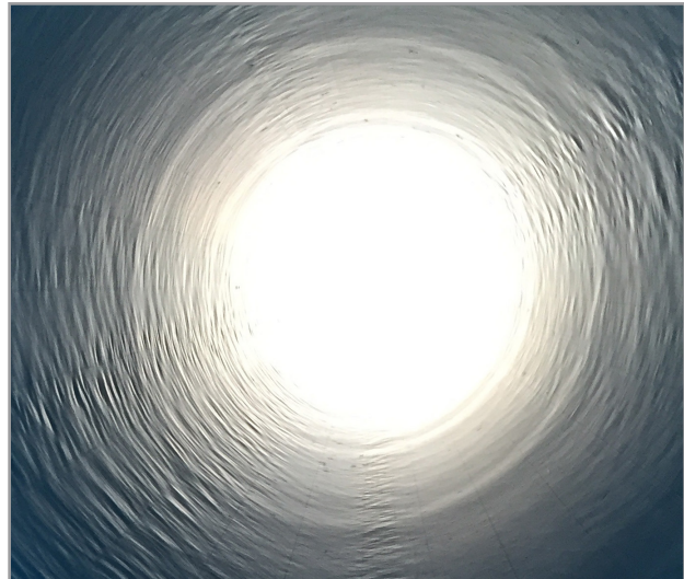
Acceptable rippling on the inside diameter of PVC pipe under natural lighting conditions
